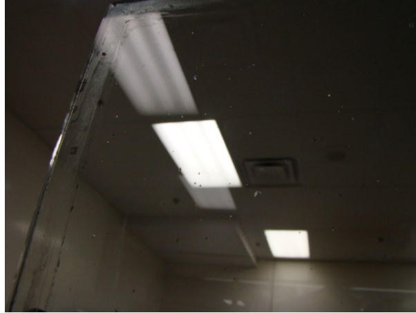
Figure 1 Weld Splatter on Glass
